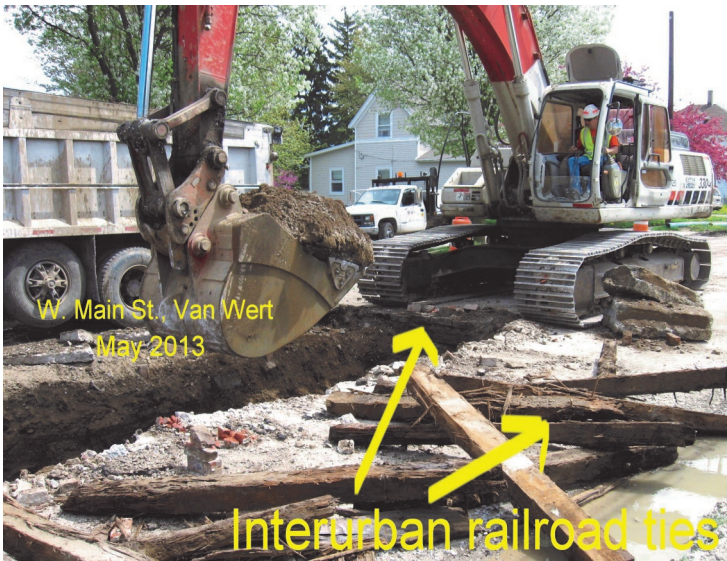
Photo: W. Main St., Van Wert, May 2013-Interurban RR ties being removed from the middle of the street.
